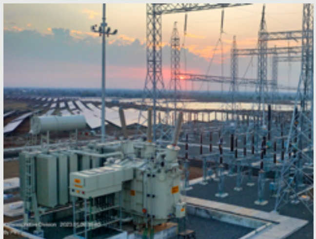
220 kV Switchyard, Khandwa
